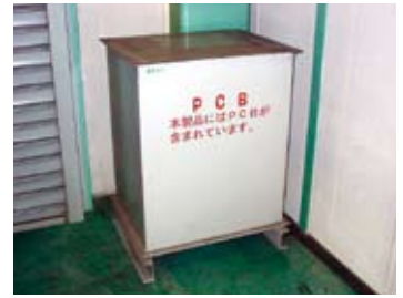
Container for waste polychlorinated biphenyls (PCBs) at Kyoto Frame Plant
